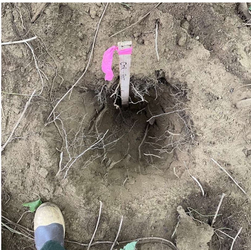
Photo 6. A view of the air excavation at deck footing 2, which is 17 feet to the east of tree 1813. No structural roots were found.
